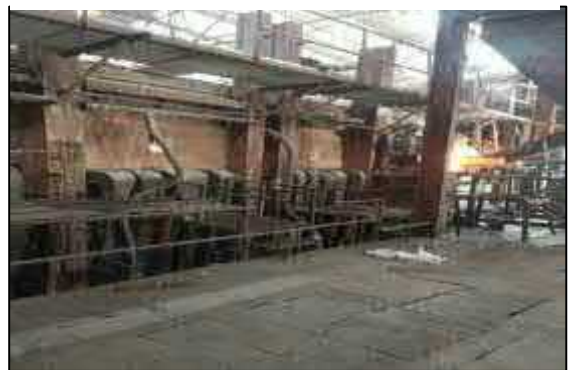
Figure 7: Typical Tank Furnace – Sample Photo
